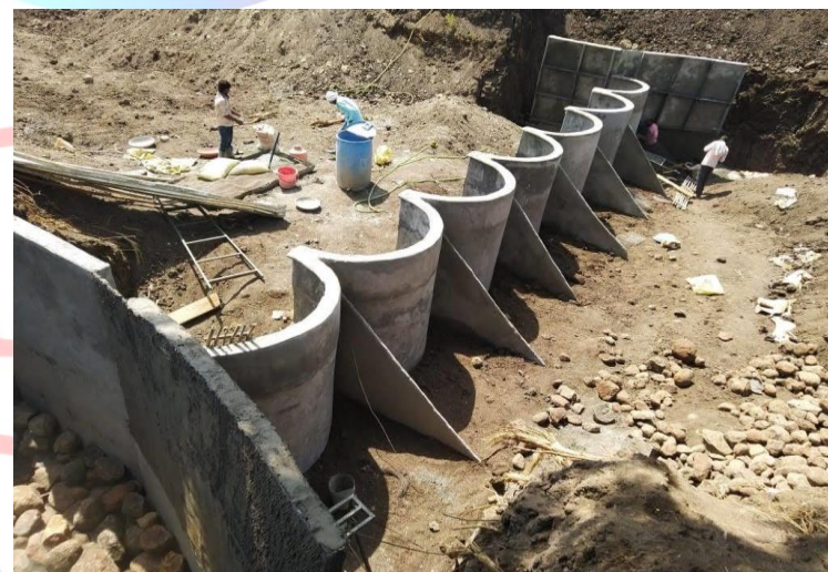
Water Storage / Dam
